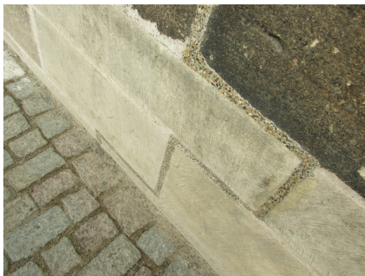
Figure 4.7: Dilatation joint and contrast between old and new blocks [Toesca, 2014].
