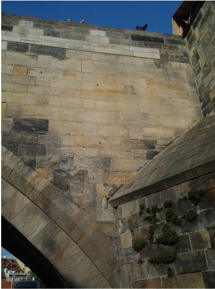
Figure 4.8: Visible vertical cracks in the southern breast wall of arch No. XI near pillar No. 10.
