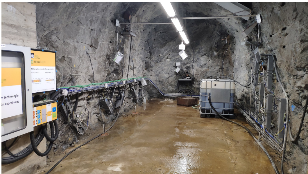
Figure 5.5: Installation of physical models in the test chamber ZK-3S at Bukov URF, heated models on the left and unheated models on the right [Svoboda et al., 2019a].
