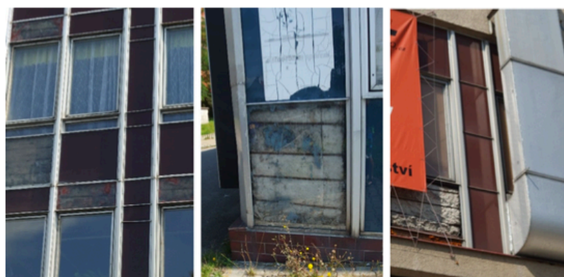
Fig. 2. Details of aluminium and glass curtain wall on building from 1970s on various buildings in Pilsen, Czechia.
