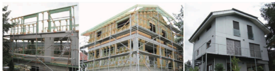
Figure 14. Construction of the family house from CS3. Left: structure of the second floor and timber frames of the third floor. Centre: complete structural system, prepared for installing a
