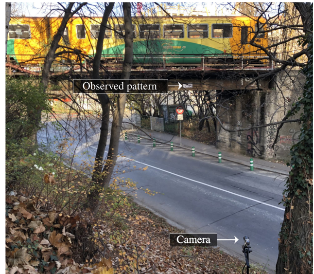
Fig. 10 Real-time measurement of a steel bridge deflection under a 40 t train engine using RTCorr
