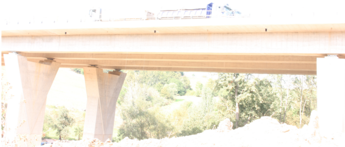
Figure 2.2: Image of the monitored bridge overexposed due to changes in the sunshine intensity over the course of the day.
