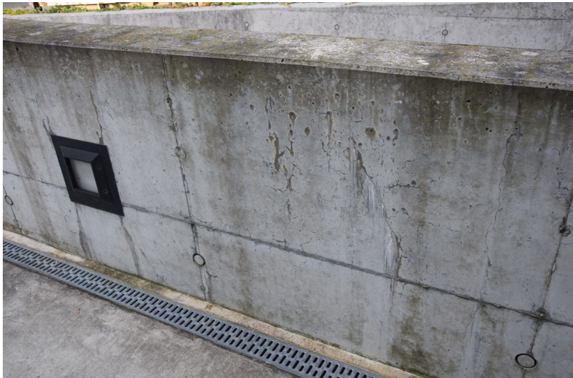
Figure 3: Cracks in a concrete pavement after \sim 17 years and in a parapet wall after 13 years.
