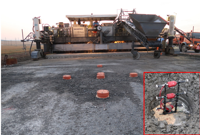
Figure 23: Vibrating wire gauges under protective covers. Detail at one assembled location.
